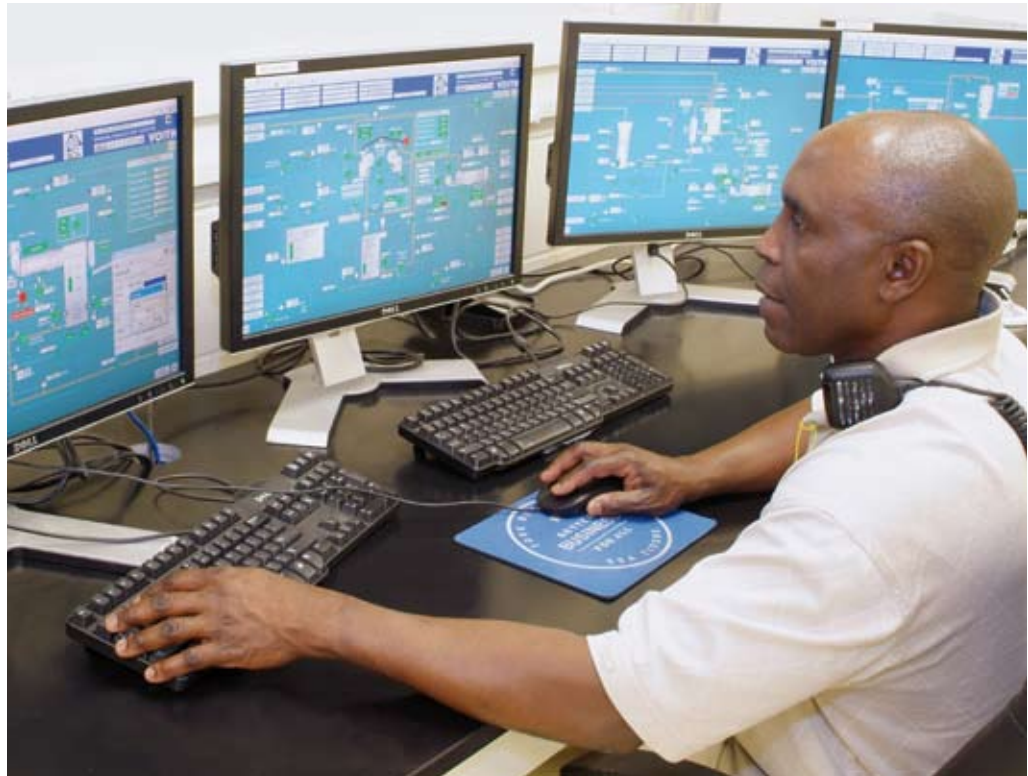
View of control room: Visualization of process control system for the de-inking facility.
