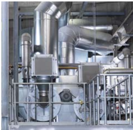
Ventilation technology for MCB-Dryer.
