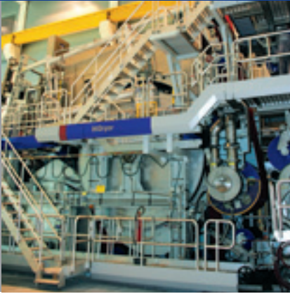
HiDryer facility at the Voith Paper Technology Center (PTC)
