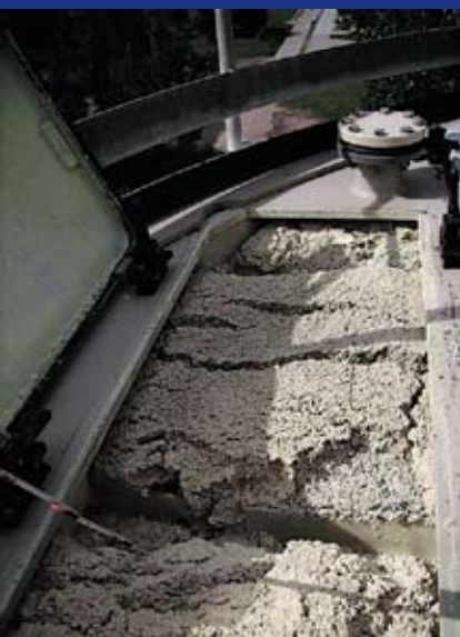
Weir blockage at the reactor head
