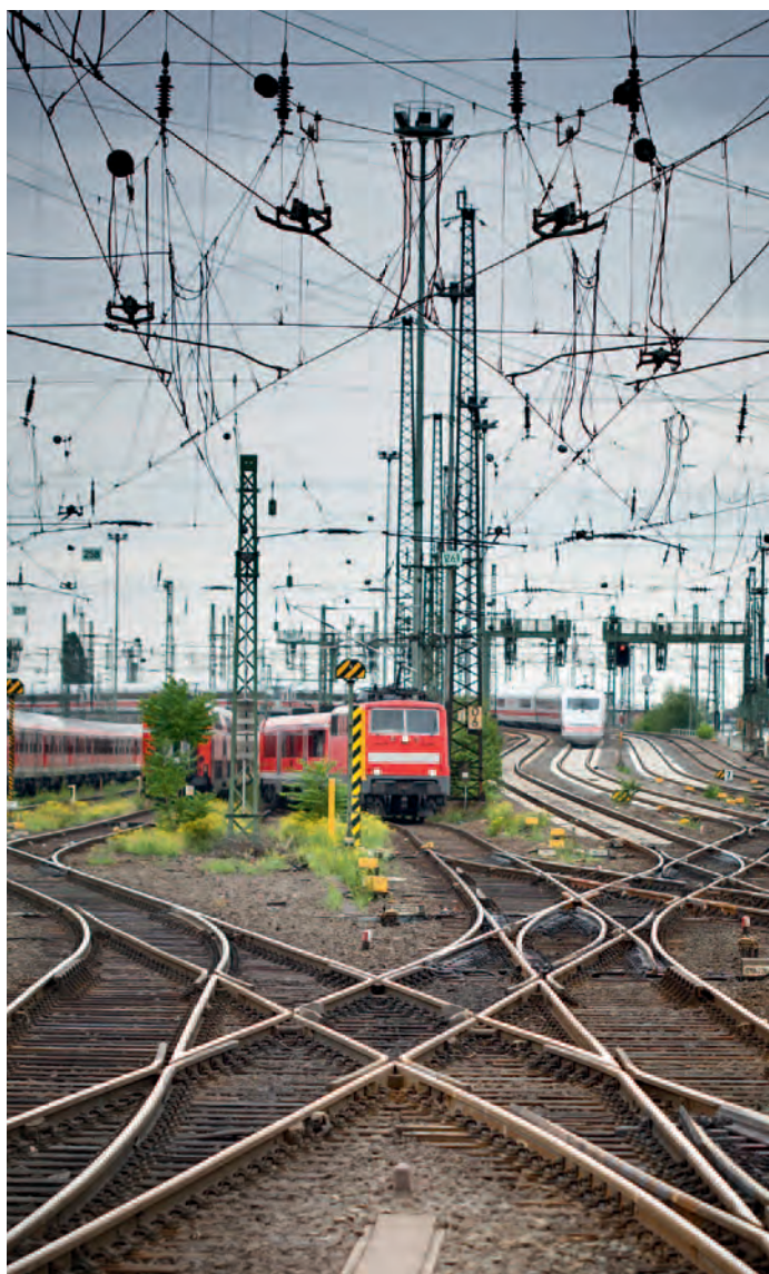
Deutsche Bahn is the single largest consumer of electricity in Germany and requires its own special network.
