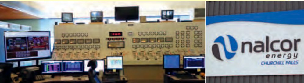
After about 40 years of service, CF(L)Co decided to replace control systems at Churchill Falls. Electronic automation will enable optimized operation thanks to more available information.
