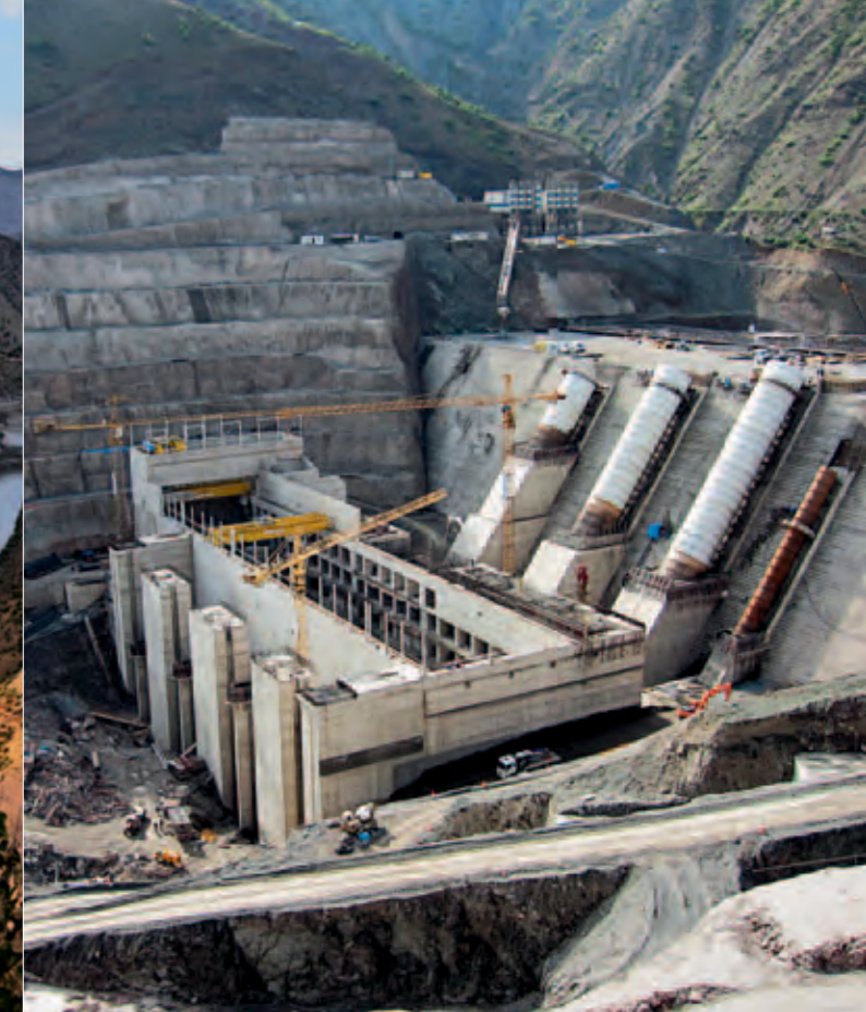
Beyhan I is the first of four hydropower plants in this area of the Murat river. Voith Hydro is fitting the plant with three generators.
